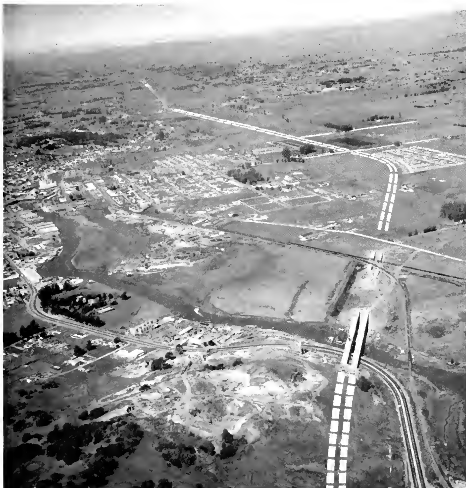
Route of the freeway bypass of Petaluma where operations are under way on two contracts for the structures and roadwork for the new facility
